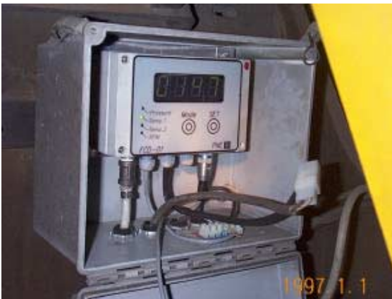
Figure 16 - Logger Unit and Enclosure
